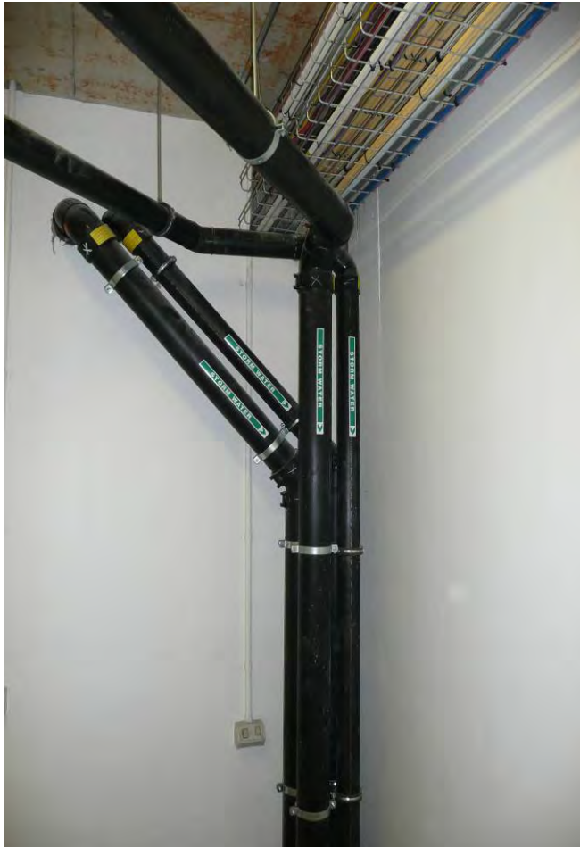
Gravity collection system in basement from multiple sources
