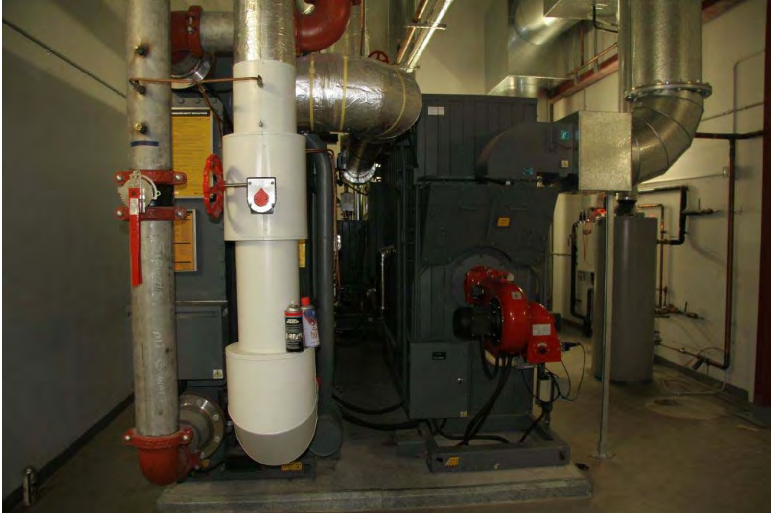
Base load gas powered generator
