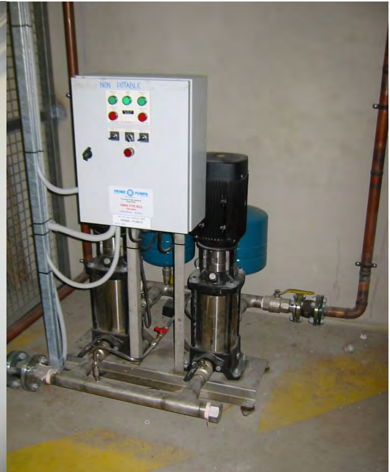
Rainwater pumps in basement
